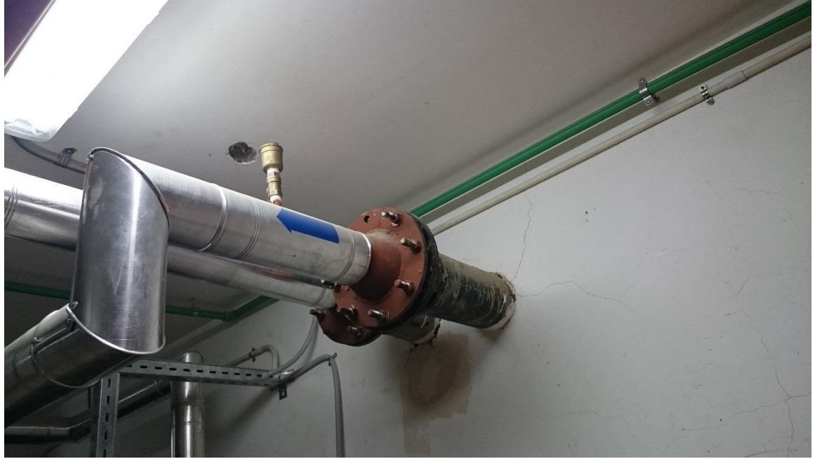
Figure 12: Ceiling Suspended piping from the pool to the Heater room
