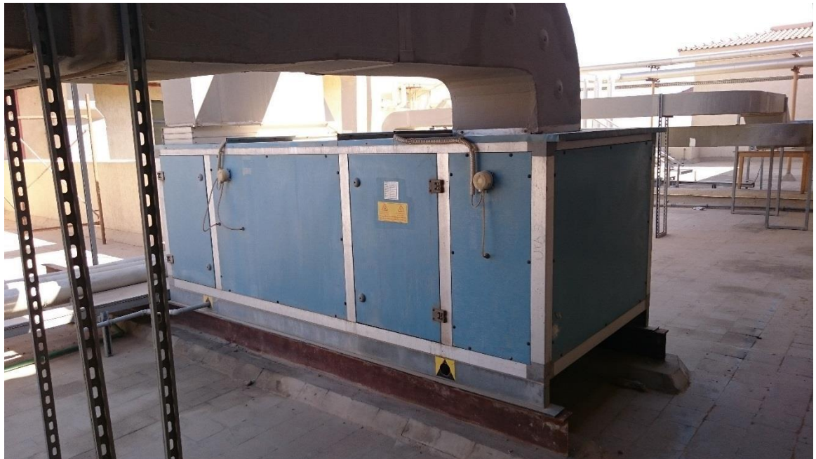
Figure 20: Air Handling Units (AHUs)
