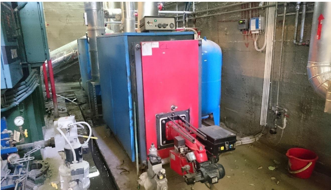
Figure3: Diesel Heater for the LTC
