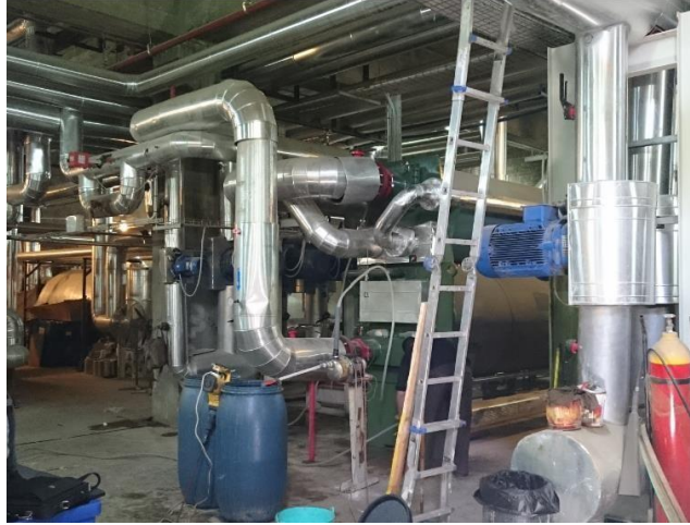
Figure 4: Small Tonnage Chiller (STC) and piping
