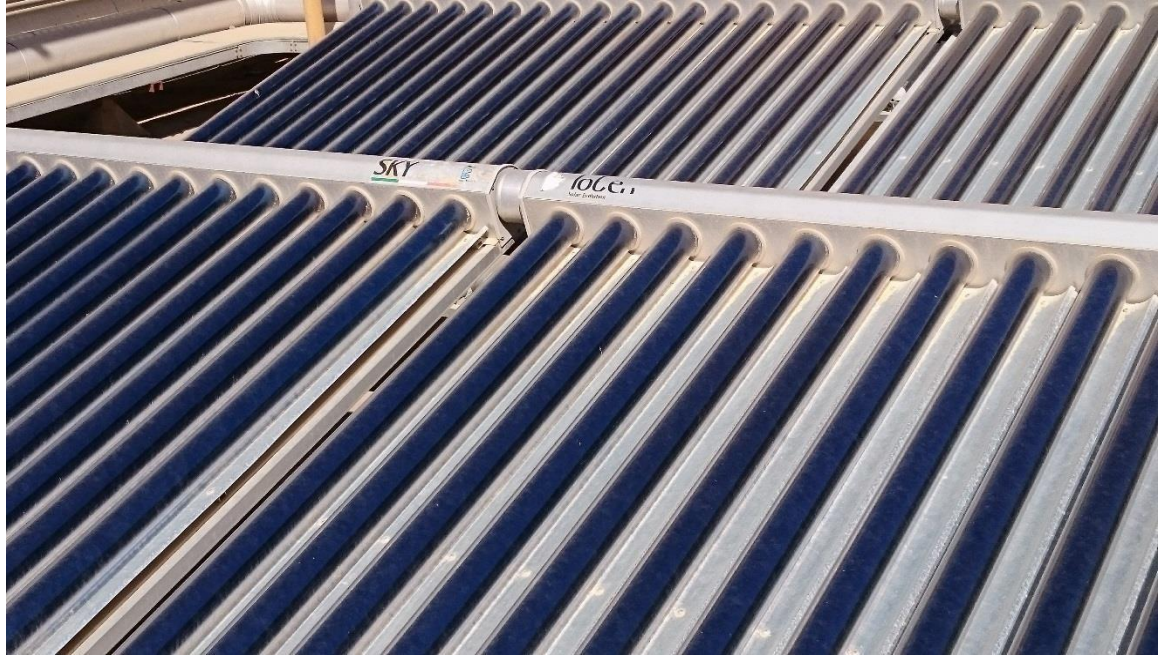
Figure18: On Roof Solar Pannels
