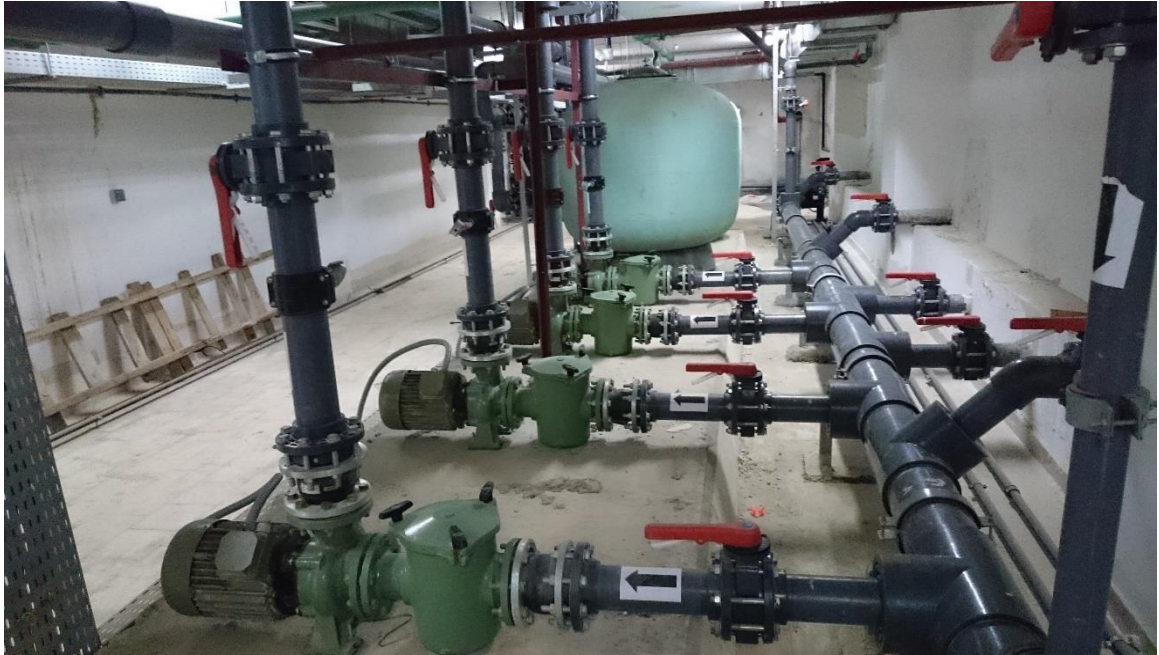
Figure 41: Swimming Pool Heater Pumps
