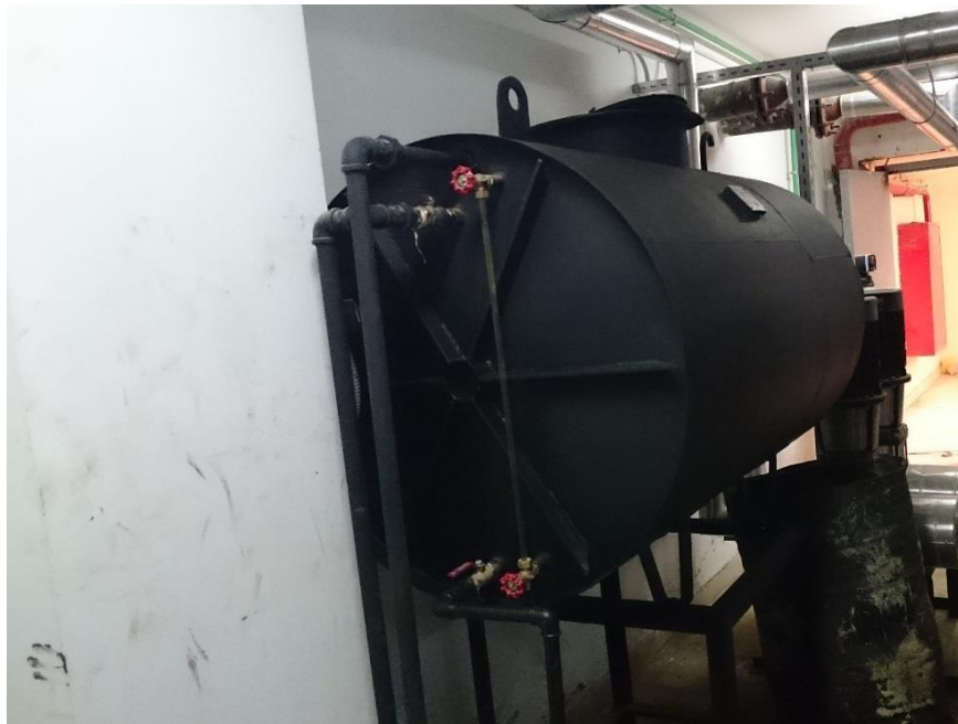
Figure 11: Diesel Container to run the Heater
